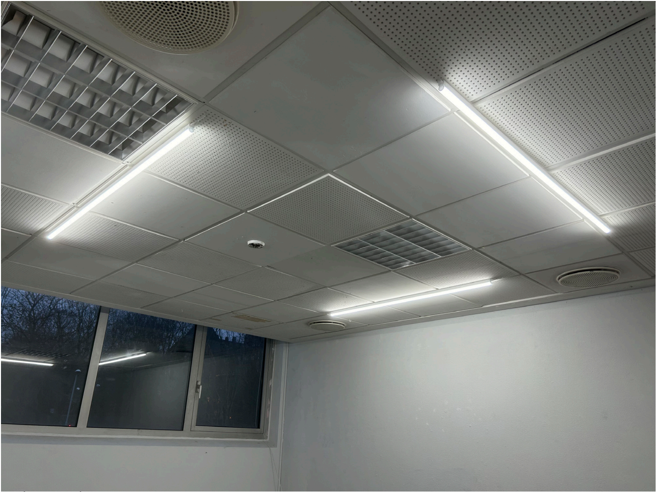
Lights in ceiling
